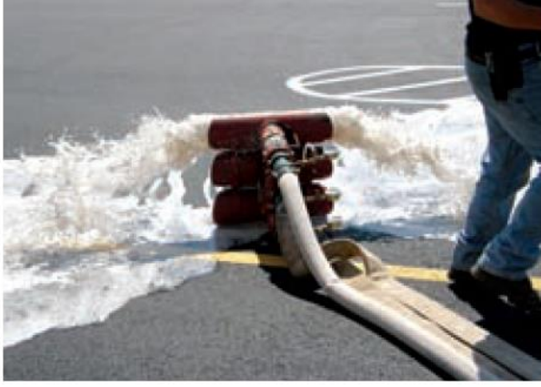
EXHIBIT II.4.21 Fire Hose Connected to Hose Monsters. (Courtesy of Aon Fire Protection Engineering)
