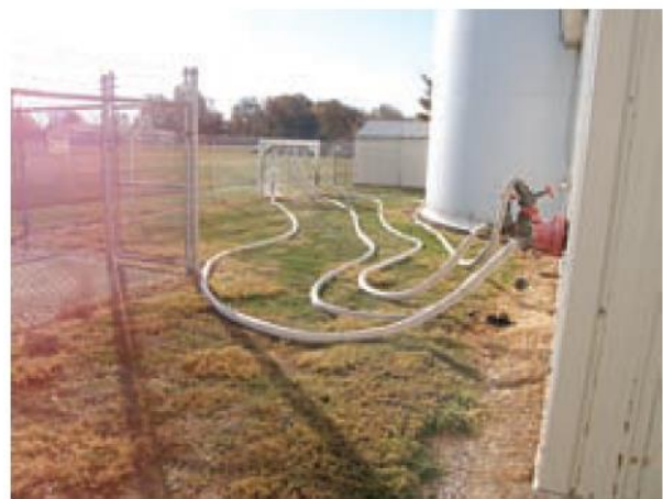
EXHIBIT II.4.20 Test Header with Hose Attached. (Courtesy of Aon Fire Protection Engineering)
