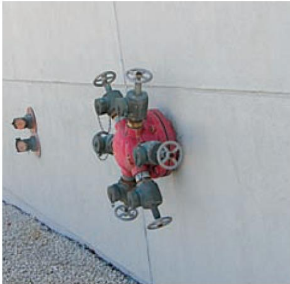
EXHIBIT II.4.19 Test Header. (Courtesy of Aon Fire Protection Engineering)
