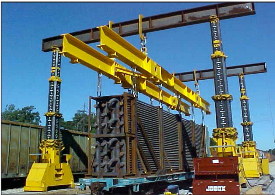
Figure 5.6-3 Pair of Hydraulic Gantries with Header
