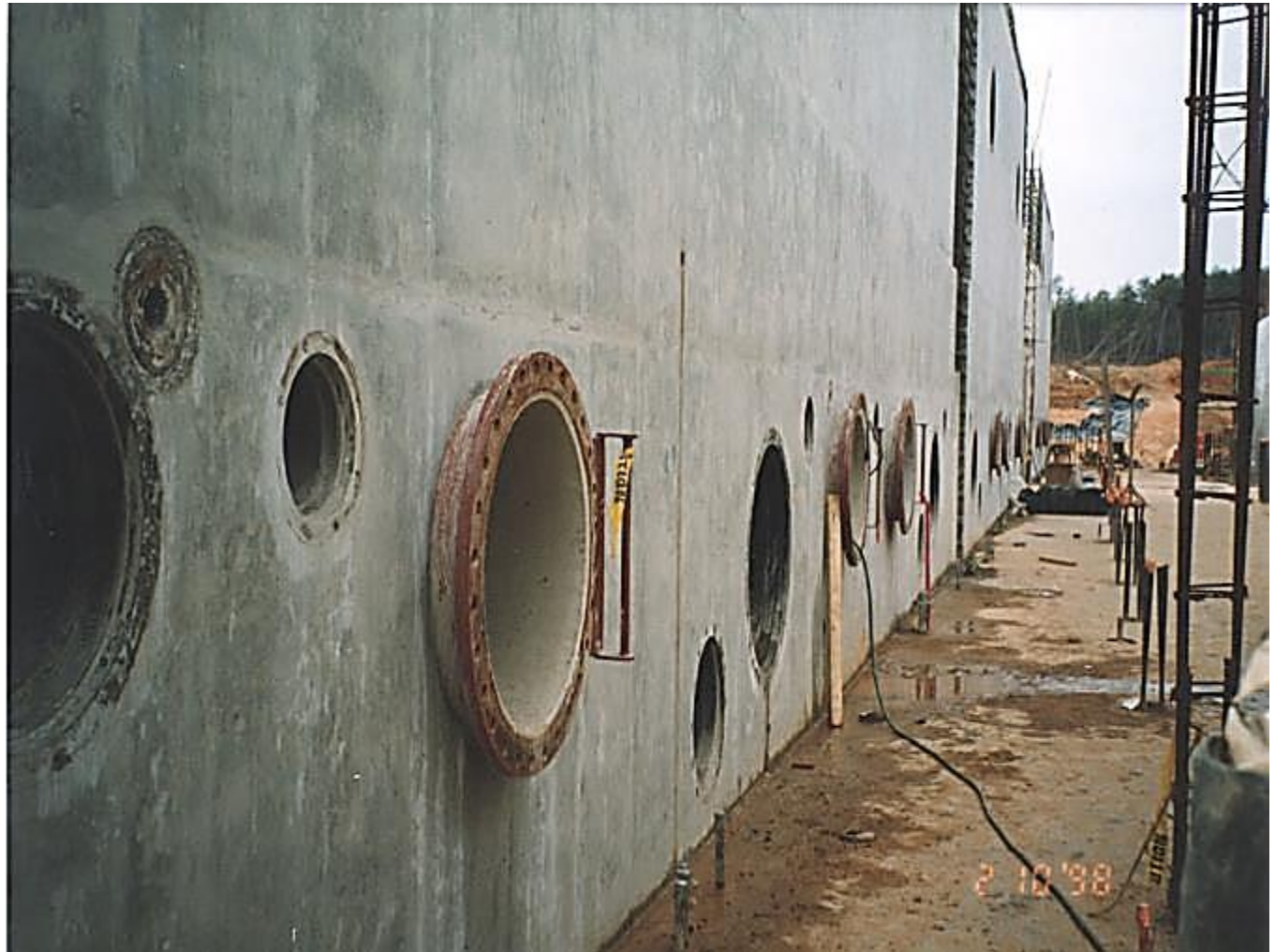
Enclosed Water Tanks
