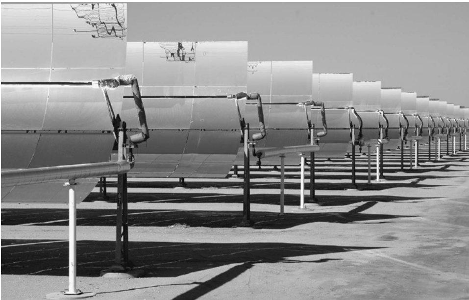
A solar energy generating facility in California's Mojave Desert. Renewable energy, including solar, wind, hydroelectric, biomass, and geothermal power, makes up only about 13 percent of U.S. energy production, but the percentage is growing every year. (iStockphoto.com)
