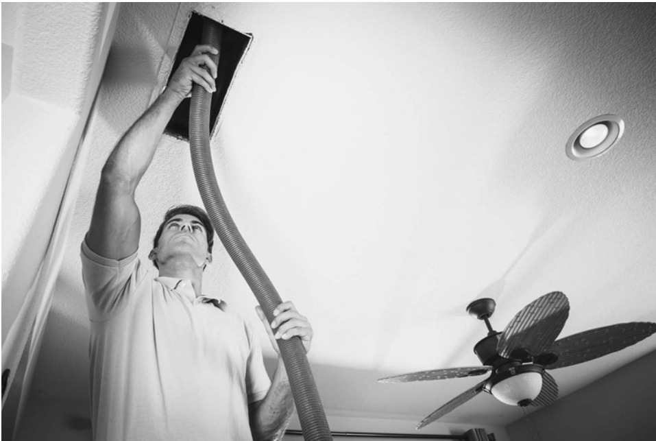
Air duct cleaning inside a home. Because people spend up to 90 percent of their time indoors, maintaining a healthy indoor environment can help prevent illness. (Bill Oxford/iStockphoto.com)
