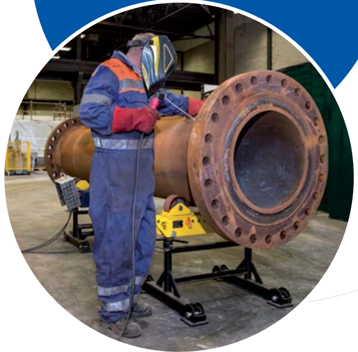
After: Rollers in position to allow operator maintain good posture while welding pipe
