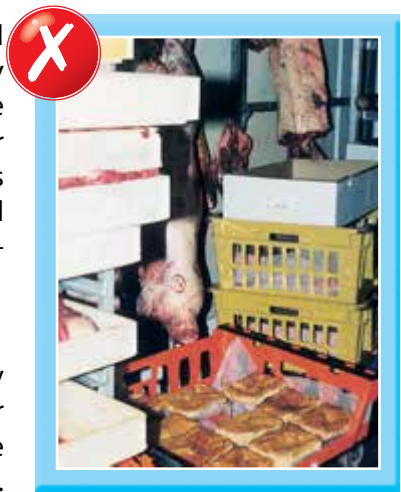
Ice build-up on the cooling unit
