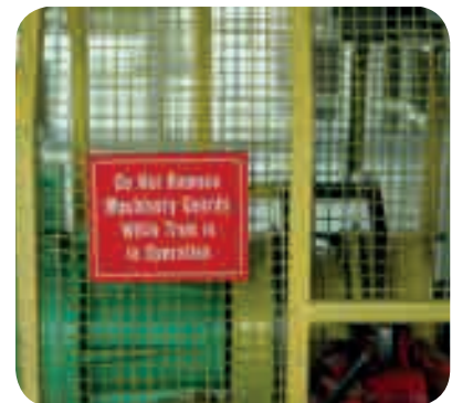
Guards reduce the risks from machinery hazards
