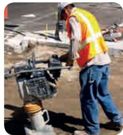
This job involves vibration exposure to the hands that must be assessed and controlled
