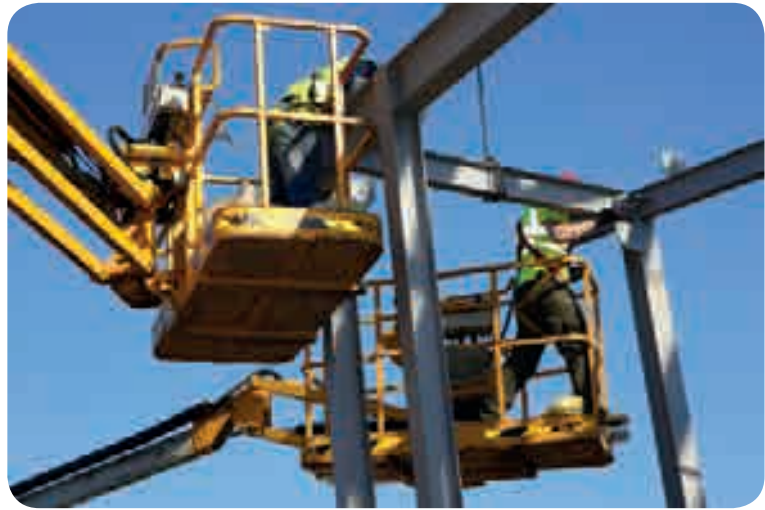
Steel workers use MEWPs to gain access to a structural steel that is being lifted into place. Note the use of full body harness despite being in an enclosed cradle
