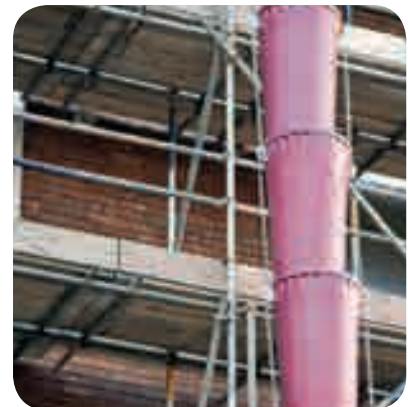
An independent tied scaffold with guardrails and toeboards. Note the debris chute for safe disposal of rubble
