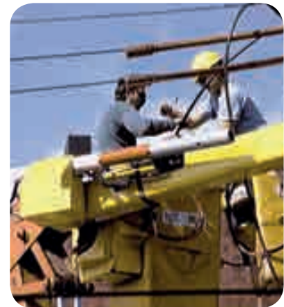
Working near overhead power lines
