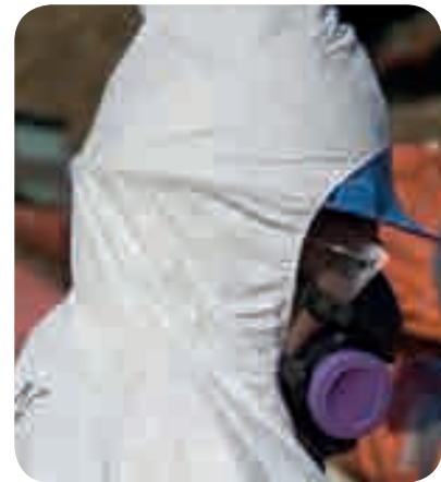
A worker wears a half-mask respirator to seal asbestos lagging around a pipe
