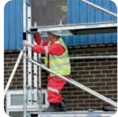
A worker gains entry to the top work platform of a tower platform of a tower scaffold through an internal trapdoor. Note the ladder built into the side of the frame. Note also the rakers or outriggers
