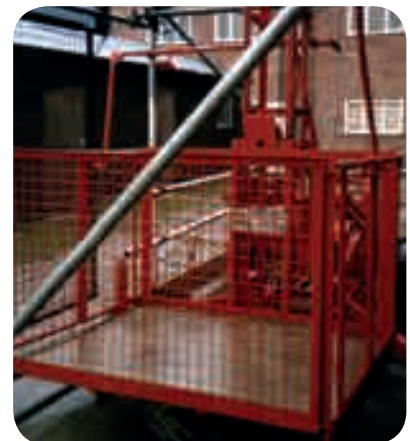
A material hoist for moving materials up and down a scaffold during roof work
