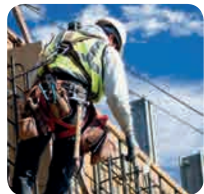
A worker using fall arrest equipment. Note the full body harness with lanyard attached at the back
