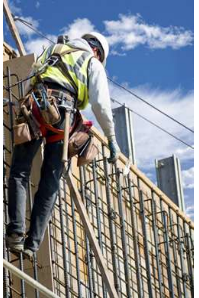
A worker using fall arrest equipment. Note the full body harness with lanyard attached at the back.
