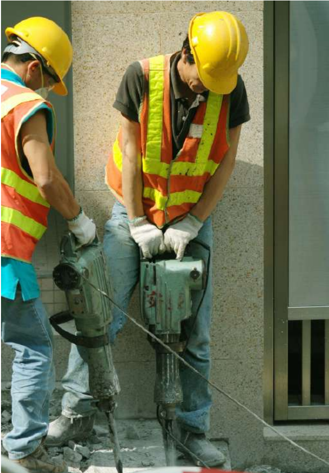
Use of jackhammers or concrete breakers; note the use of PPE, but the apparent absence of hearing protection
