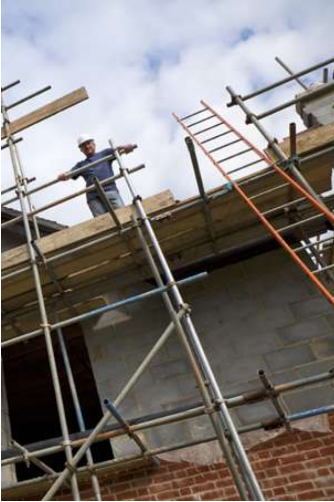
Ladder used to gain access to a scaffold platform. Note how the ladder extends well above the stepping off point and how it has been secured to the scaffold
