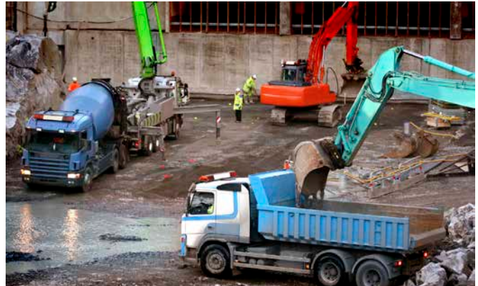
Movement of vehicles and heavy plant is a common site hazard that must be closely supervised
