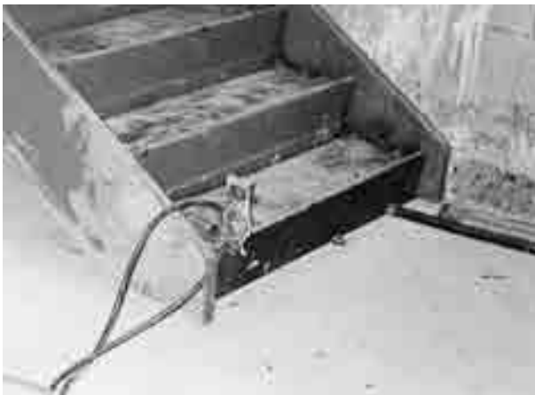
FIGURE 7.4 Grounding for an arc welder
