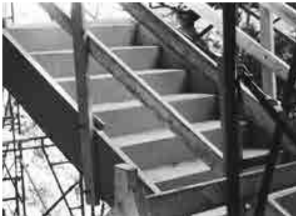
FIGURE 8.42 Stair pans filled with wood
