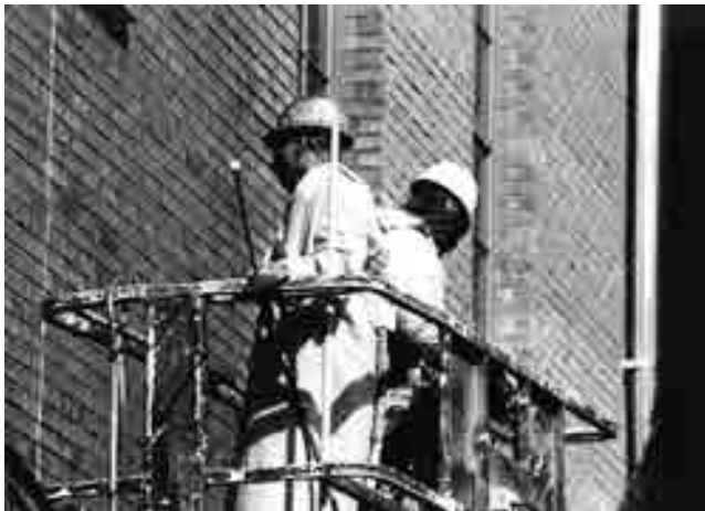
FIGURE 9.21 Cleaning buildings with high pressure chemicals may generate hazardous mists or vapors
