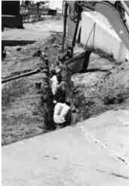
FIGURE 7.34 Workers in an unprotected trench
