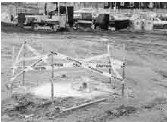
FIGURE 7.6 A barrier marked with caution tape
