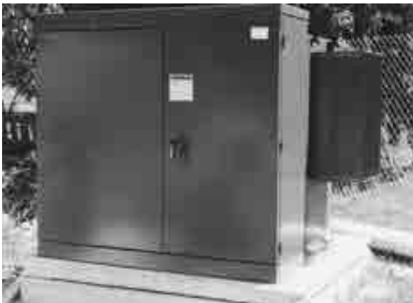
FIGURE 7.25 Electrical enclosure accessible to qualified persons
