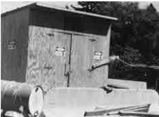
FIGURE 7.31 Typical dog house as a barrier from electricity for unqualified persons
