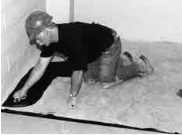
FIGURE 9.25 Floor adhesives may contain coal tar pitch volatiles
