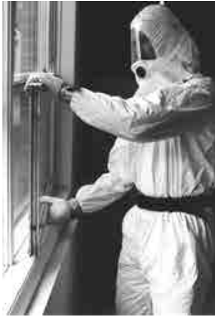
FIGURE 10.24 Powered air-purifying respirator used by a window contractor for potential lead dust exposure
