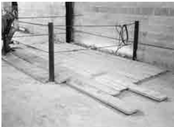
FIGURE 7.51 Covered and guarded floor opening ( Note: although it cannot be seen, “Hole” was painted on this cover. )
