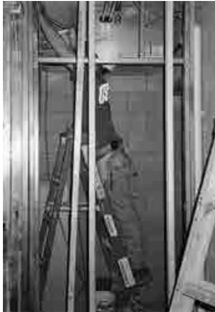
FIGURE 11.9 Electrician in a work position which causes him to have to raise his arms above his shoulders
