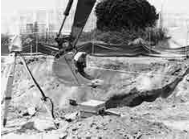
FIGURE 1.8 Unsafe act — worker riding in bucket
