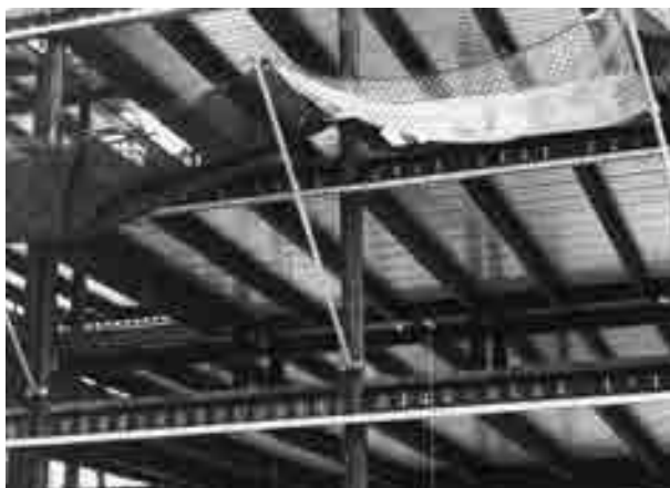
FIGURE 7.47 Example of a perimeter safety net
