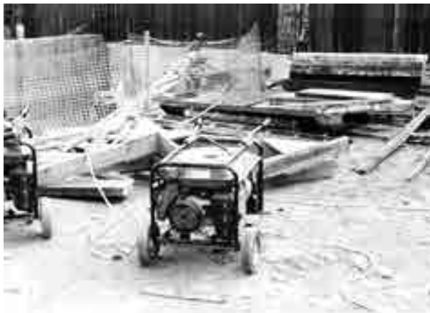
FIGURE 7.29 Example of portable electrical generator
