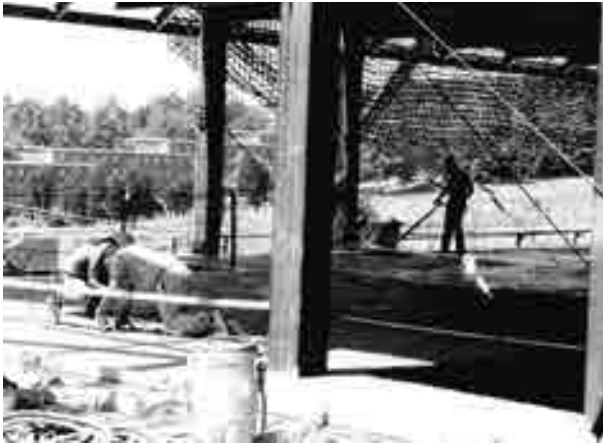
FIGURE 11.15 Workers performing hand troweling while worker in the background uses a mechanized trowel
