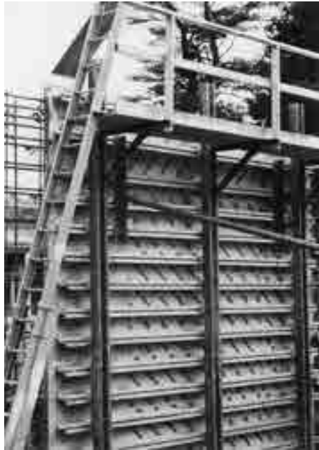
FIGURE 7.46 Guardrail system on formwork
