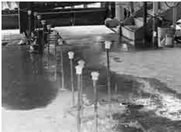
FIGURE 7.10 Protected rebar to guard against impalement
