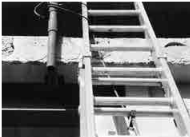
FIGURE 8.2 Extension ladder secured and three rungs above the landing area
