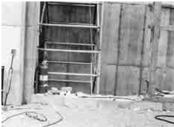
FIGURE 7.52 Typical fire extinguisher on a construction site
