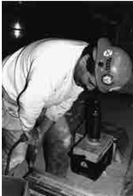
FIGURE 9.3 Positioning of tools may cause ergonomic hazards
