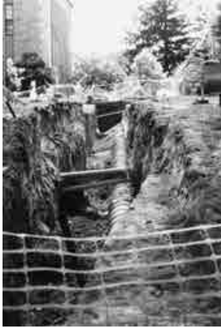
FIGURE 7.35 Unsupported trench and underground installations
