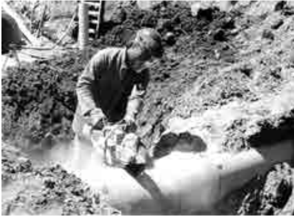
FIGURE 9.18 Cutting pipe could generate dust containing asbestos
