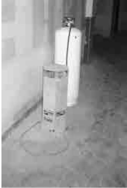
FIGURE 7.59 Example of a temporary heater
