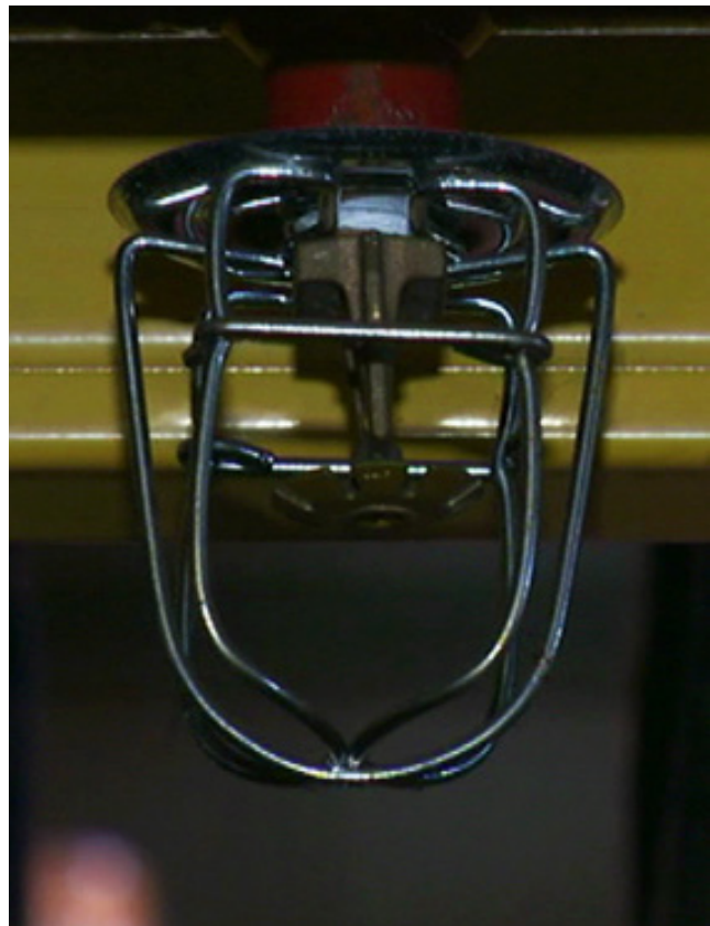
Figure 10.9: Sprinkler head in warehouse racking
