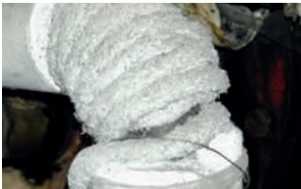
Asbestos lagging rope and lagging
