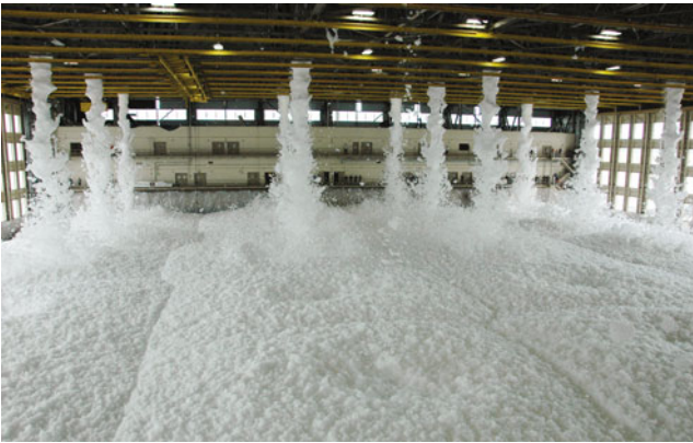
Figure 17.6 Foam emanating from outlets Source: Elgin Air Force Base.
