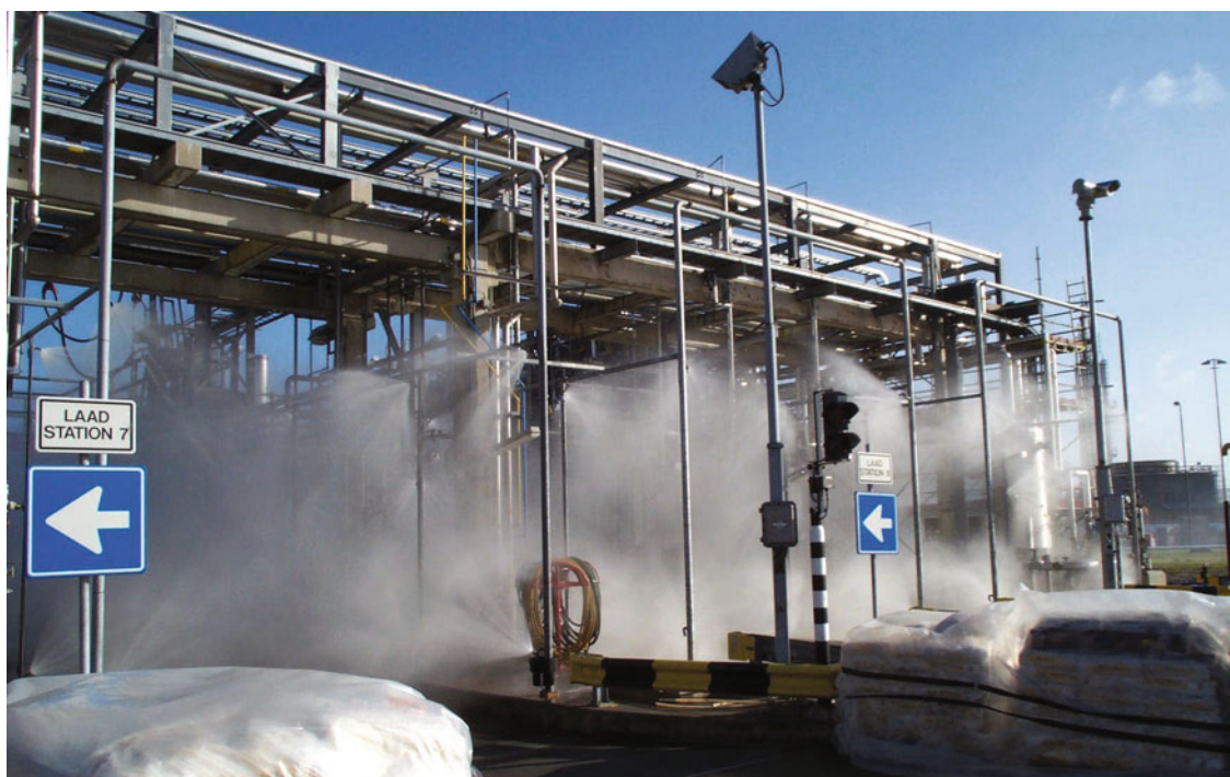
Figure 9.2 Fire deluge system Source: Frontline Fire International.
