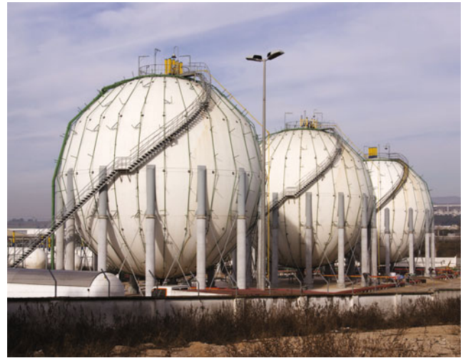
Figure 17.14 Spherical tanks with fire protection system Source: iStock.
