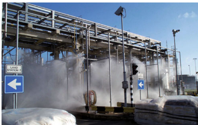
Figure 13.2 Fire deluge system Source: Frontline Fire International.
