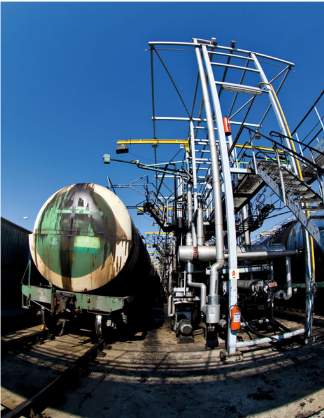
Figure 20.6 Loading arrangements for rail tankers Source: Dreamstime.
