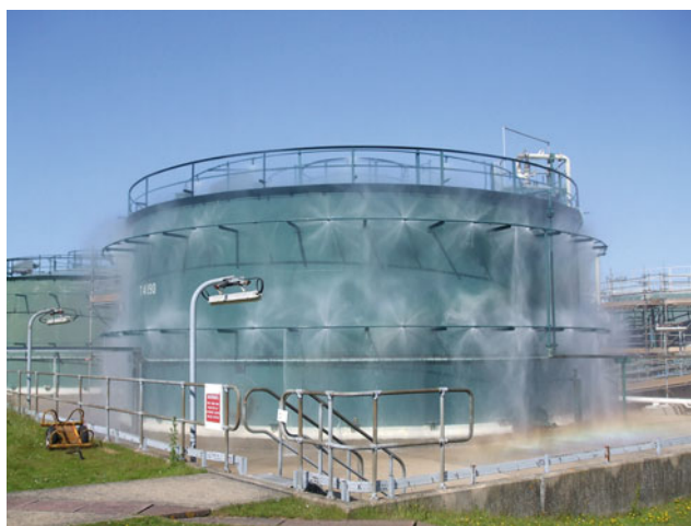
Figure 17.11 Tank spray system in action Source: Martin Wall – Shutterstock.
