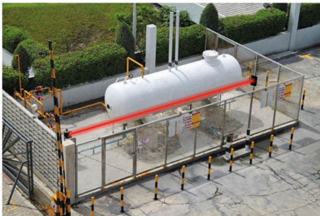
Figure 17.2 Infrared beam detector in situ Source: Dreamstime.
