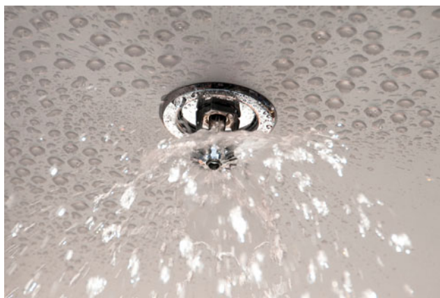
Figure 17.5 Sprinkler head in action Source: iStock.
