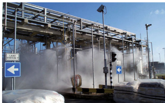
Figure 17.3 Fire deluge system Source: Frontline Fire International.
