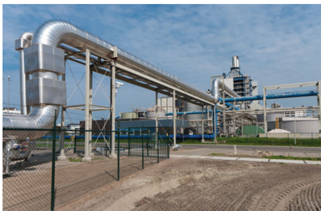
Figure 14.6 Pipes going over bund
