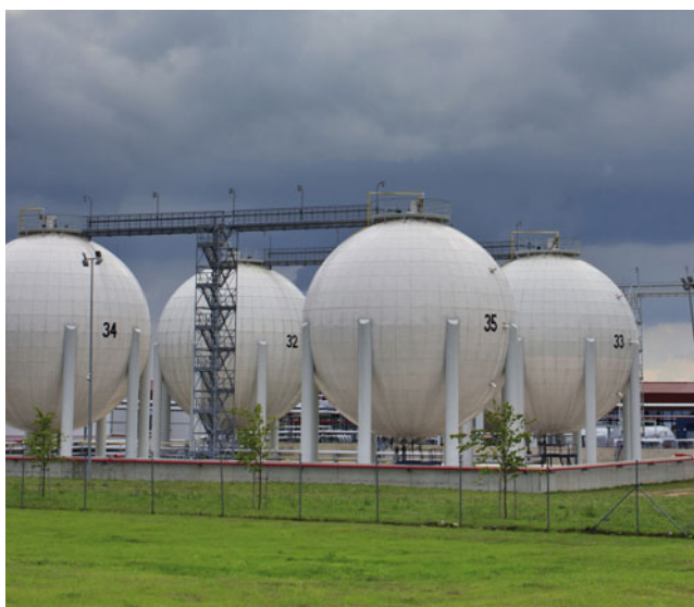
Figure 14.9 Spherical storage tanks Source: Dreamstime.
