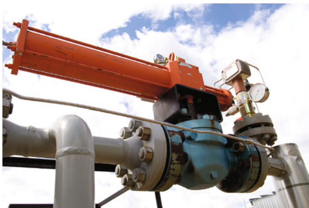
Figure 13.1 Emergency shutdown valve Source: iStock.
