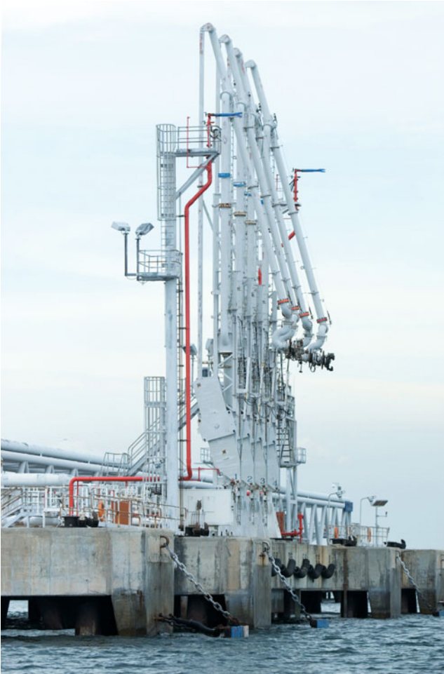
Figure 19.6 Oil loading arms
