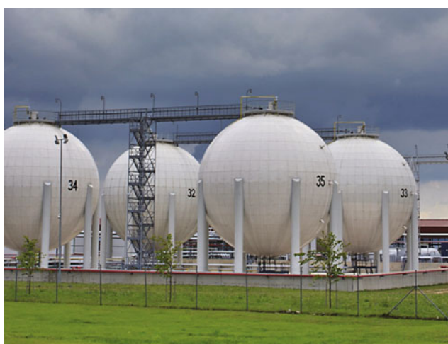
Figure 17.12 Spherical storage tanks Source: Dreamstime.
