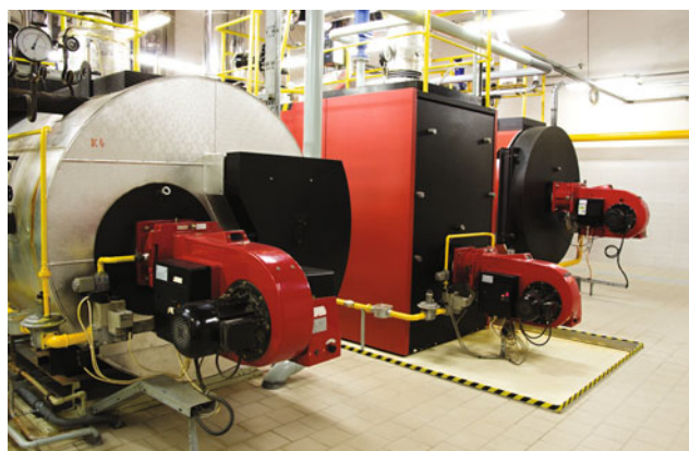
Figure 16.1 Boilers Source: Dreamstime.
