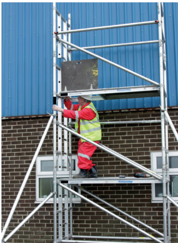
A worker gains entry to the top work platform of a tower scaffold.
