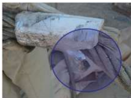
Cracked and Split Ferrule
