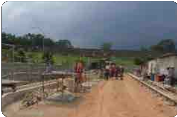
Figure 13: Location where the worker was stationed on the day of the incident.
