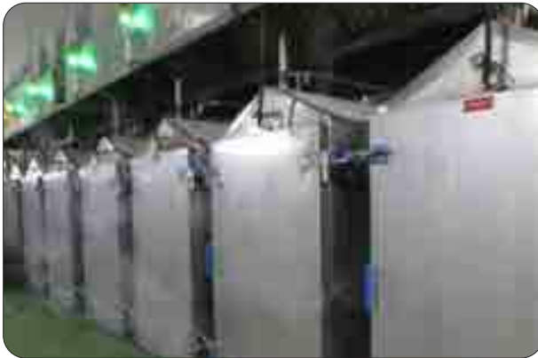
Figure 12: The worker was tasked to work in the vicinity of the above food steamers in the food processing factory.
