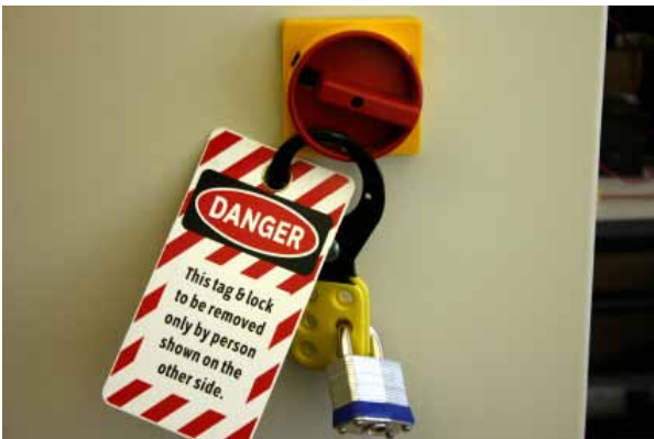
Lock out/tag out systems provide warnings and safeguards
