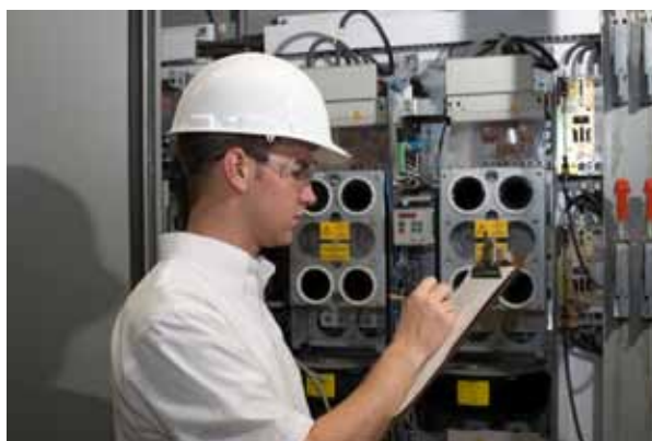
Certain tests and inspections will be required before start-up
