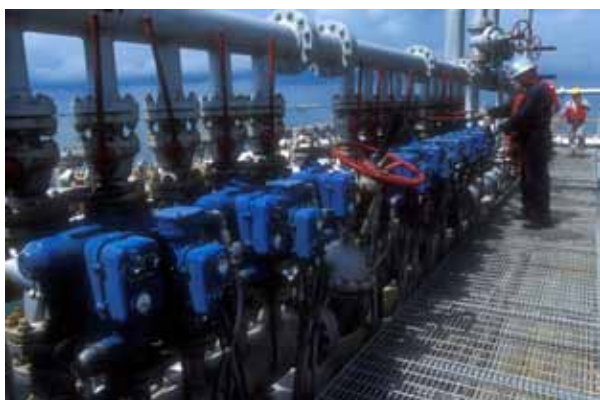
The most critical items of plant should be inspected regularly
