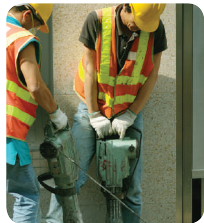
Vibration exposure may lead to risk assessment
