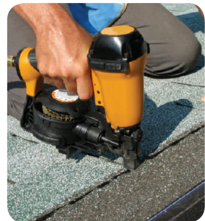
Equipment must be selected appropriately
