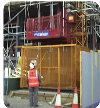
Electric hoist moving load
