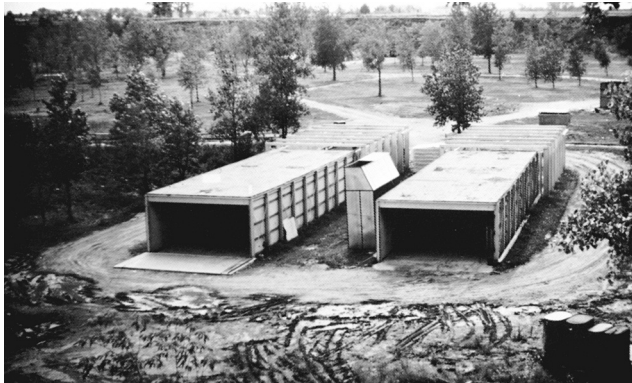
FIGURE A.38.3.2(a) Overall View of 20 ft × 100 ft (6.1 m × 30 m) Fire Test Building from Exhaust End.
