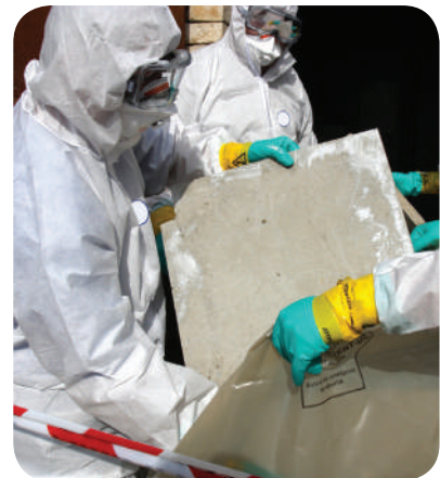
Removal and bagging of ACM Note the protective clothing and the use of RPE
