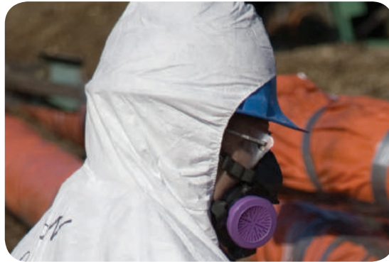
A worker wears a half-mask respirator to seal asbestos lagging around a pipe
