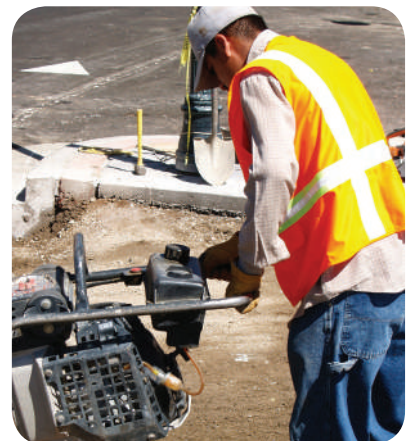
Compactors and other tools can generate a lot of vibration, which is then delivered into the hands and arms of the worker
