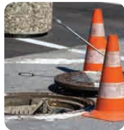
Controls and safeguards should be in place
