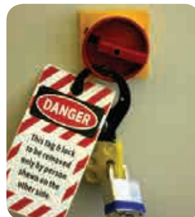
Electrical isolation as part of the permit-to-work system
