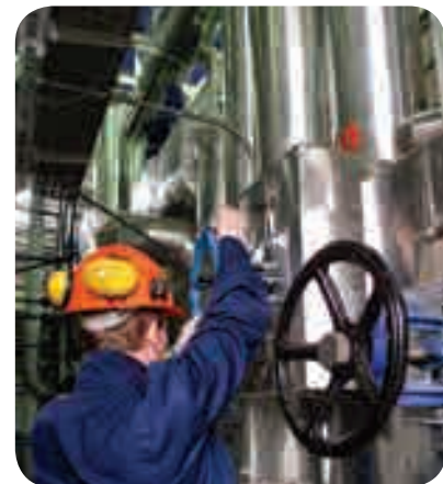
Modifications to pressurised systems
