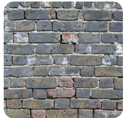
Moisture is the greatest cause of deterioration in buildings
