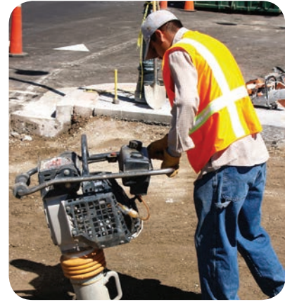
Vibration from machinery can affect structural weakness in buildings
