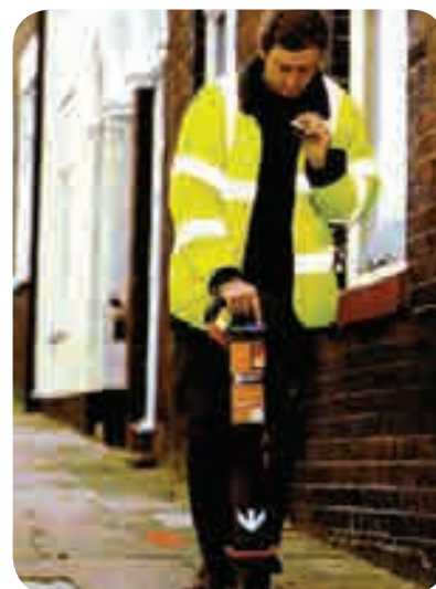
Using a cable locator Source: HSG47 Avoiding danger from underground services, HSE, 2014 ( www.hse.gov.uk/pubns/priced/hsg47.pdf )
