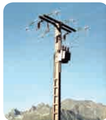
Overhead electricity lines
