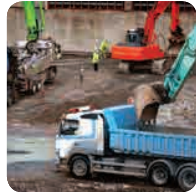
Congested sites increase the risk of collision
