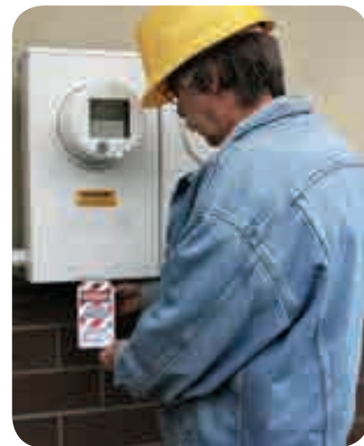
Electrician places a lock-out tag on an electrical panel
