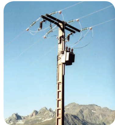
Overhead electricity lines
