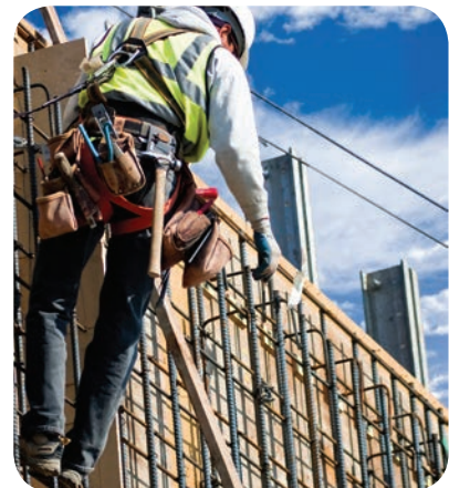
Worker using fall-arrest equipment - note the full body harness with lanyard attached at the back
