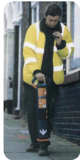
Using a cable locator Source: HSG47 Avoiding danger from underground services, HSE, 2014 ( www.hse.gov.uk/pubns/priced/hsg47.pdf )
