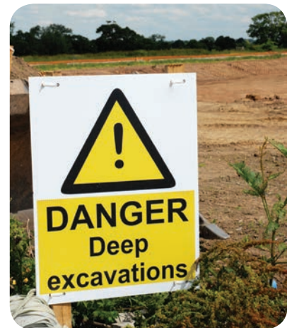
Excavations can cause fatal accidents
