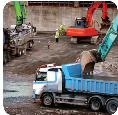
Congested sites increase the risk of collision
