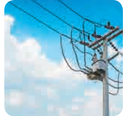
High voltage electricity
