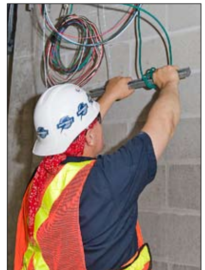
Using hand tools or spare bits of pipe eases stress to the hands while pulling wire.
