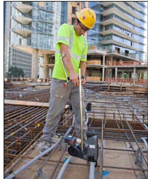
Rebar tying machines with extension arms allow workers to tie conduit while standing upright.
