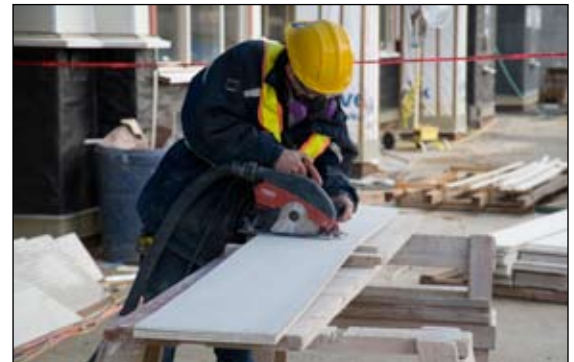
Protected worker cutting fibre-cement board using a circular saw with dust controls
