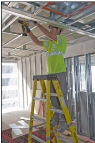
Ladders raise your body position so you are closer to the work surface.
